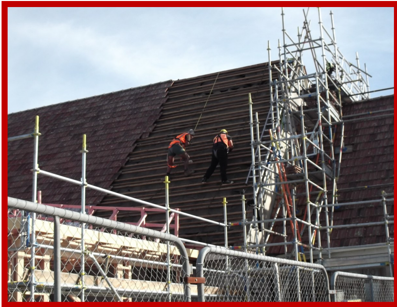
We remember when the scaffolding was up at St David's and the tiles were coming off the roof in 2017.
